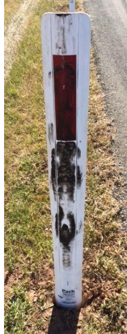
Figure 2, Post 1 after testing at 100km/h
