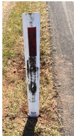
Figure 4, Post 2 after testing at 100km/h
